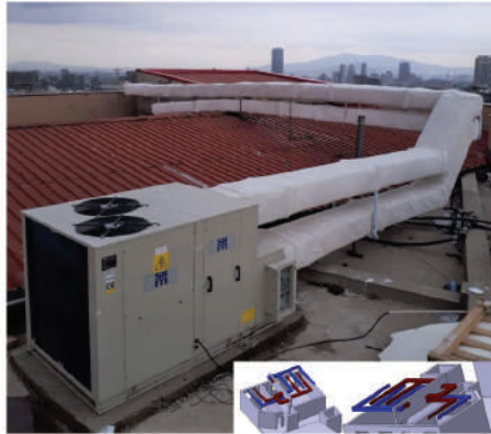
Mahbere Kidusan Television Studio – Design and Build of HVAC System
