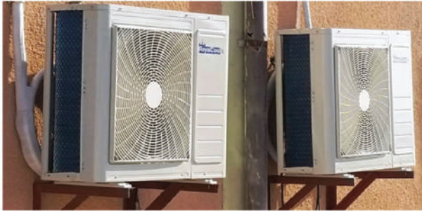
HVAC (Heating, Ventilation, and Air Conditioning)
