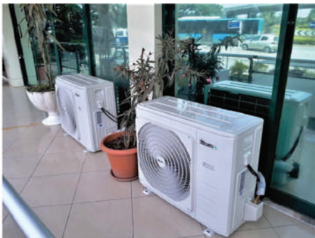
Berhan Bank Branch offices in 13 cities – HVACs
