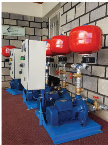
Oromia Construction Corporation – Booster Pumps
